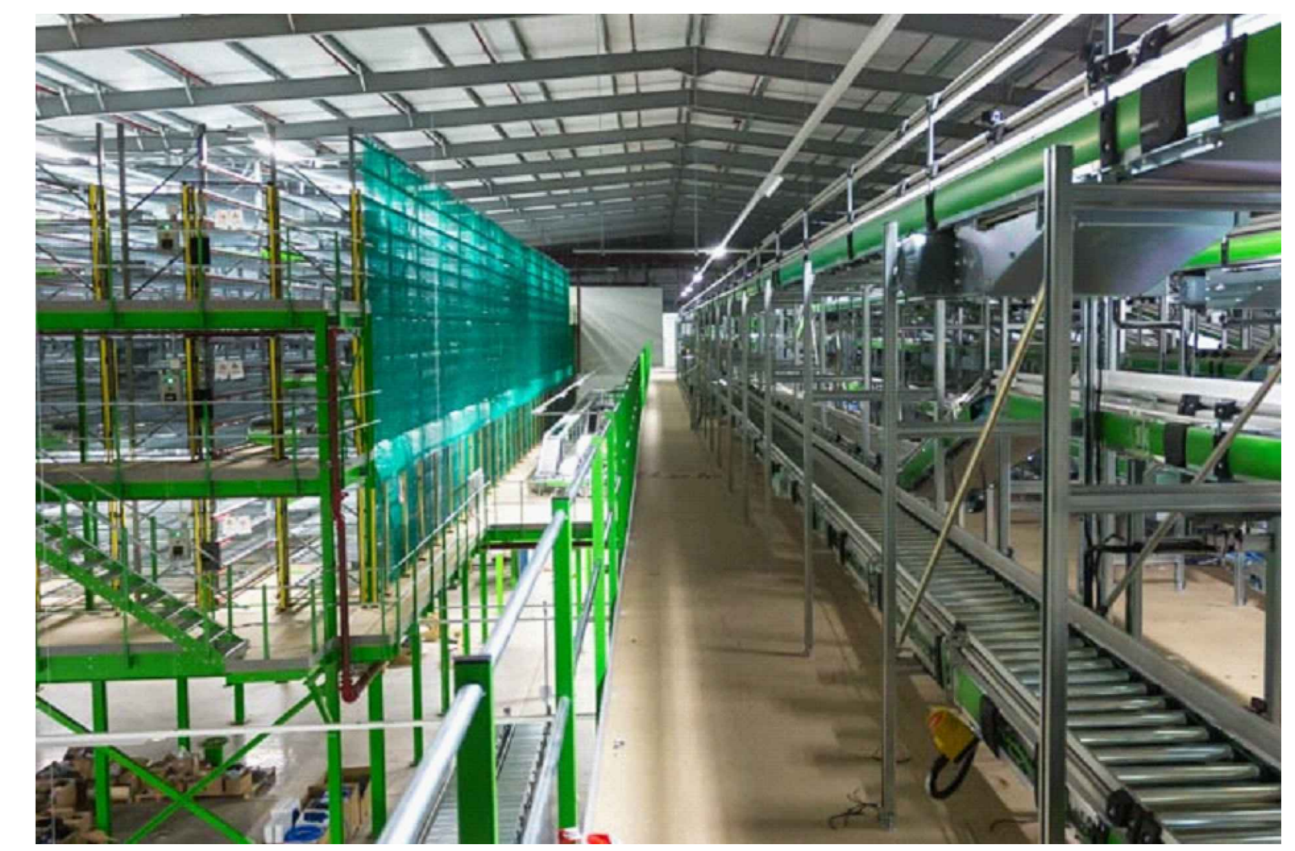
Image 2 - Mezzanine racking and automation systems
